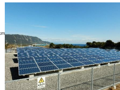
Ohara Solar Power Station
